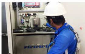
檢查SMP盤 Inspection of SMP
