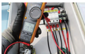
檢查JB箱-量測電流電壓 Inspection of JB - IV Measurement
