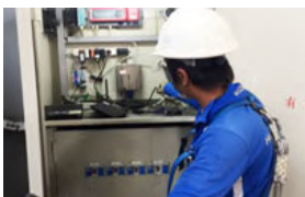
檢查SMP盤 Inspection of SMP
